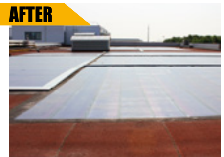
APPLICATION OF GENERAL SOLAR PV ON AN EXISTING ROOF WITHOUT DRILLING THE WATERPROOFING LAYER.
