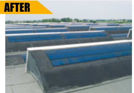
GENERAL SOLAR PV SYSTEM PLACED ON COPPELLA AND SHED
